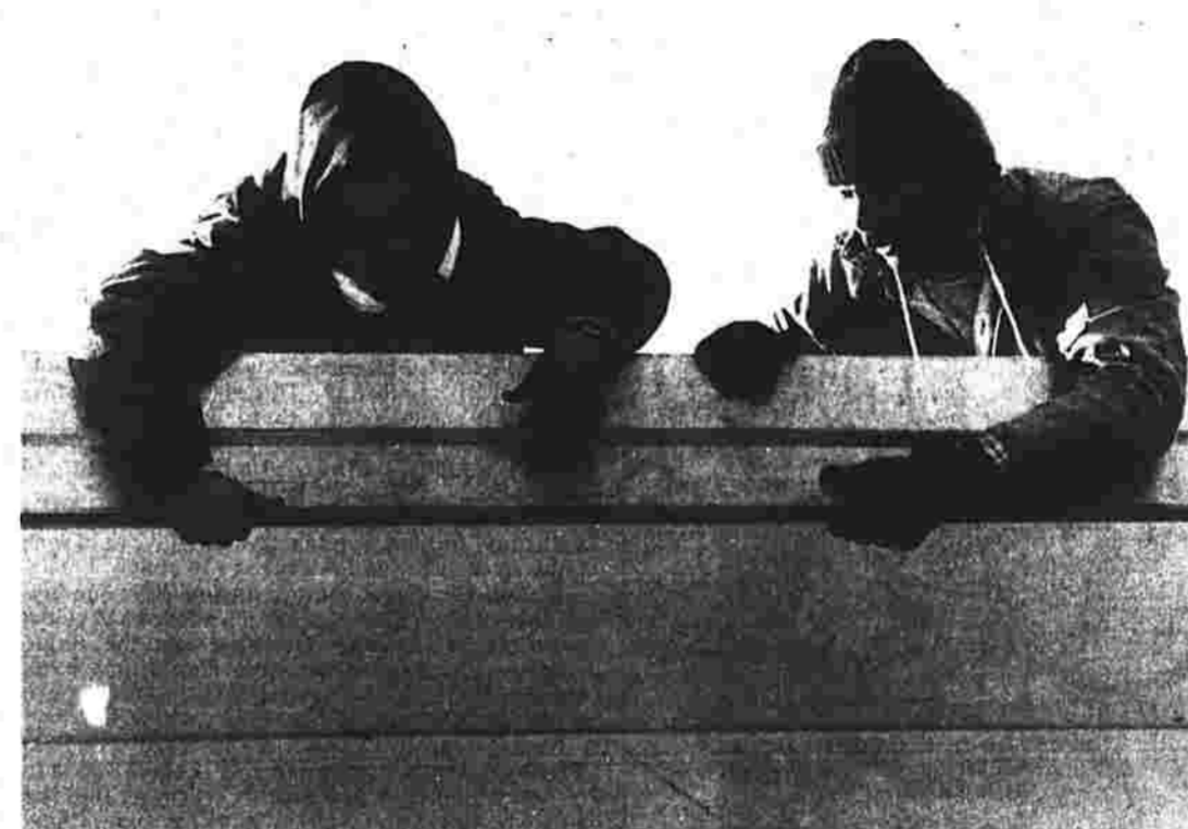
Jim McMahon, left, and Bill Copeland of Premier Roofing Co. of West Haven brave the cold Wednesday to install aluminum trim on the new roof at Bolton Center School. The $74,000 project, which began on Nov. 18, is almost complete after numerous delays caused by the weather.
